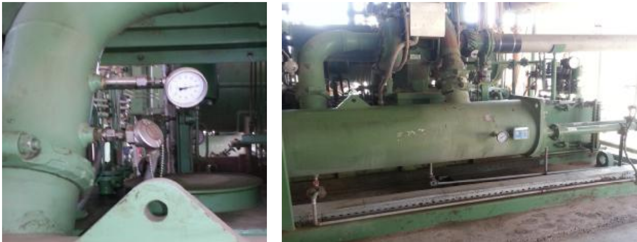
Fig. 1. Shell-and-Tube Heat Exchanger use in Practical Work (Power Generation Department in Dura Refinery).
