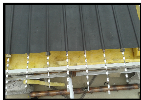
Fig. 7. A twisted strip inside riser pipe.
